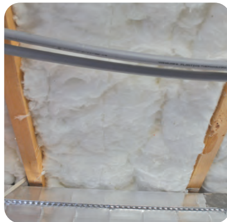
4. Batts installed with no gaps
