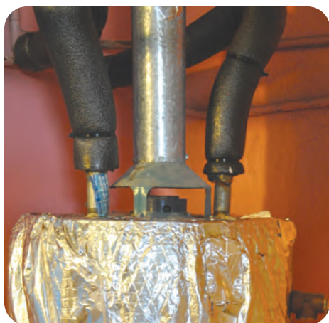
Keep insulation back at least 6 inches from draft diverter and single wall pipe
